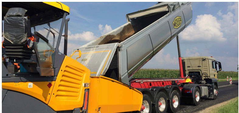
Tar surface finishing: With the tarpaulin closed, the asphalt retains its required temperature.
